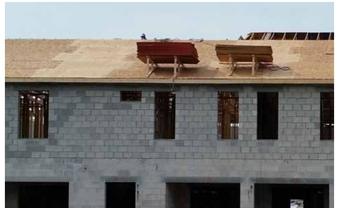
Pyro-Guard® plywood used four feet on each side of a wall to eliminate parapets. St. Petersburg, FL.
